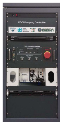
Sandia's Control System that was recently tested on the PDCI
